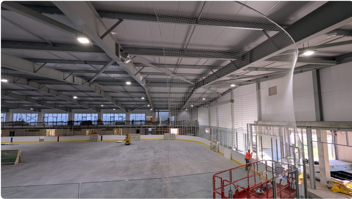
Protective netting going up above the boards at the end of the rink.
